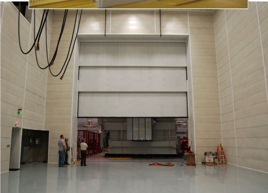
30' x 34' high NIC 47, telescoping vertical-lift door installed in Noise Barriers' 63Hz, cutoff 40' x 60' x 45' high Hemi-Anechoic Chamber.
